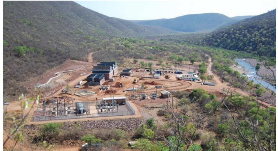
Pump Station & Electrical Sub Station
