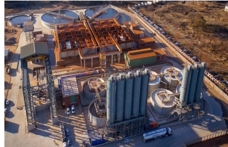
Central Basin: Completed High Density Sludge Treatment Plant
