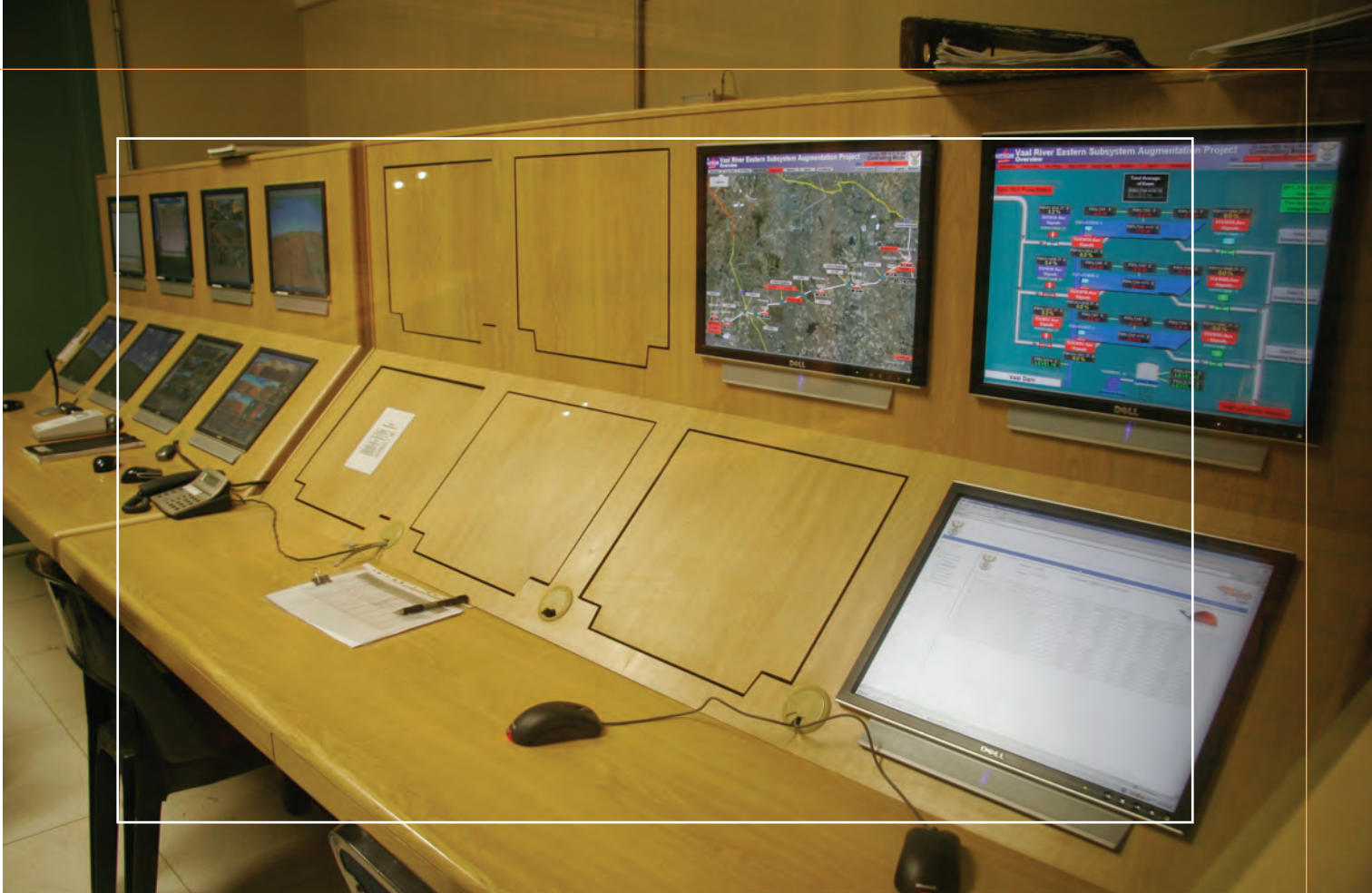
Vaal River Eastern Subsystem Augmentation Project: The project was designed to be remotely controlled from Grootdraai Dam. The control panel at the high lift pump station in Boschkop (with the entire major project components unmanned) is similar to the control panel in Grootdraai Dam, from where the operator can monitor operations in Boschkop. He can see if valves are open or closed, which pumps are running, the volume of water delivered, the level of storage dams, and if a pump trips – what the cause of the trip is
