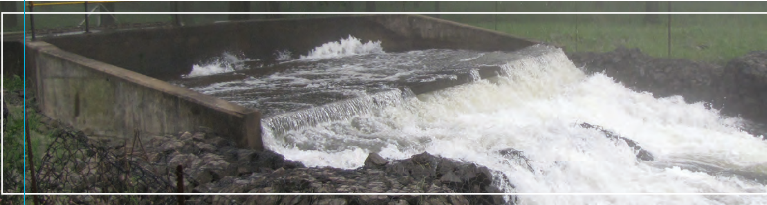
A water release structure from the existing Mooi-Mgeni Transfer Scheme into the Mpofana River (Natal midlands)
