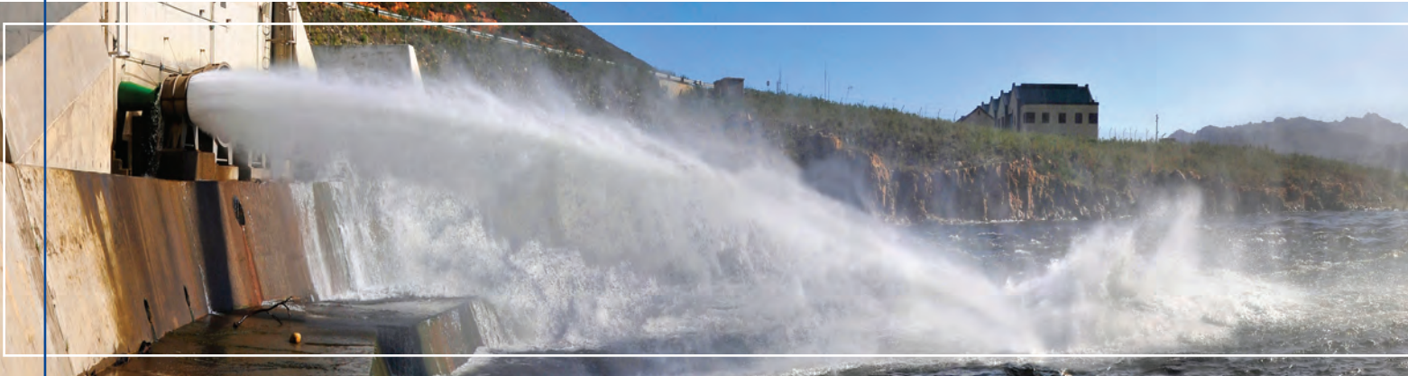
Berg Water Project: View from the sleeve valves
