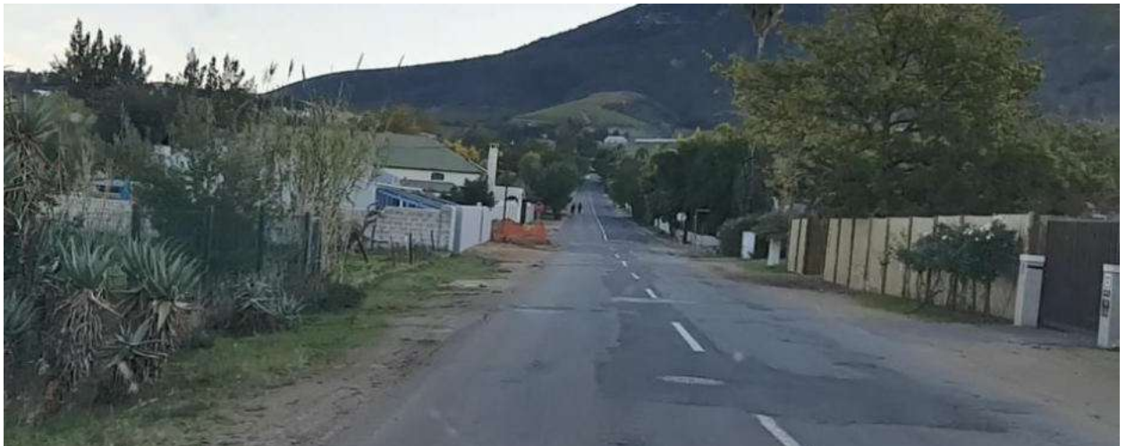
Piet Retief Street in very poor condition
