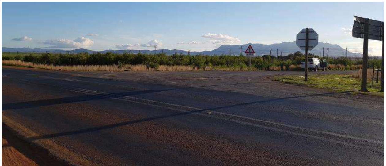
Intersection in very poor condition
