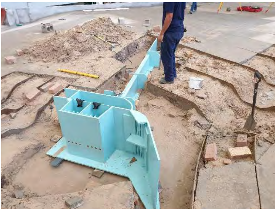
Figure 6-4: Construction of the proposed river abstraction works and weir in the physical model
