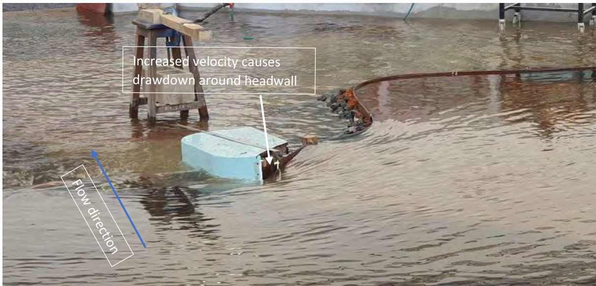
Figure 9-43: Downstream view of the RMFcc flood flowing around the berm headwall
