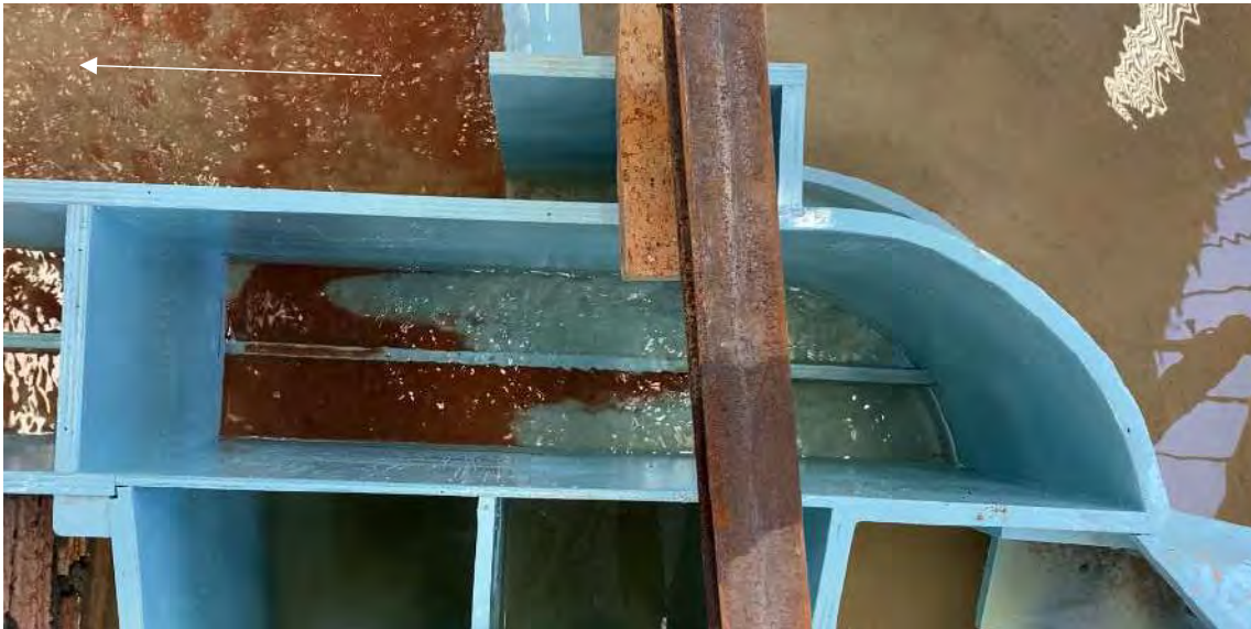
Figure 9-4: Flushing limit of the two gravel trap canals after the Q2cc (210 m 3 /s)
