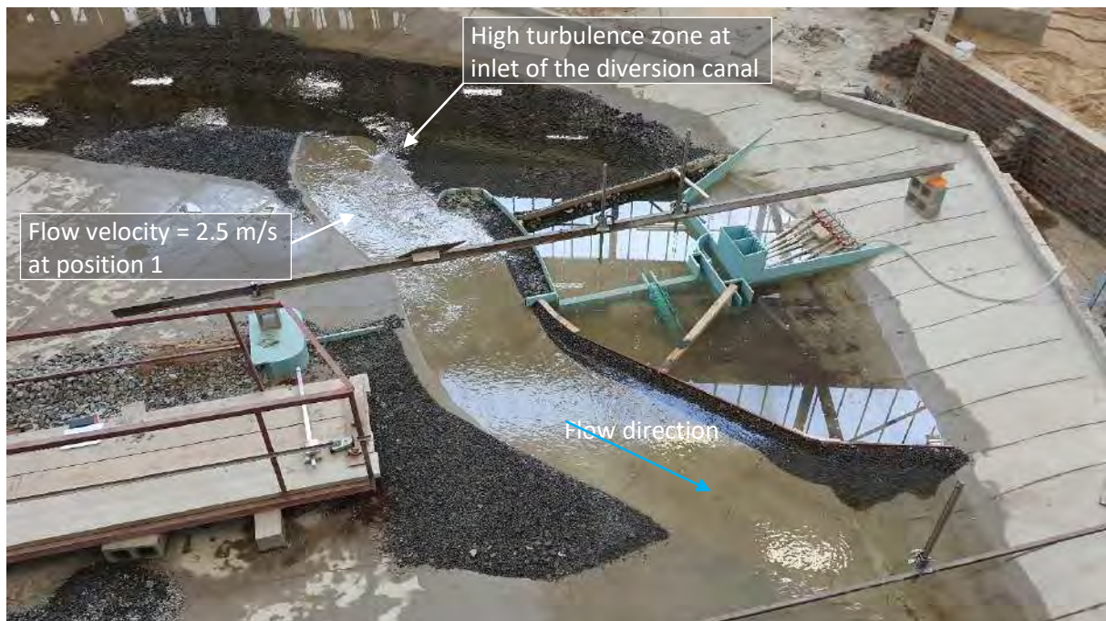
Figure 10-10: Temporary works layout of Option C for a 5-year ARI-flood (369 m 3 /s), viewed from downstream
